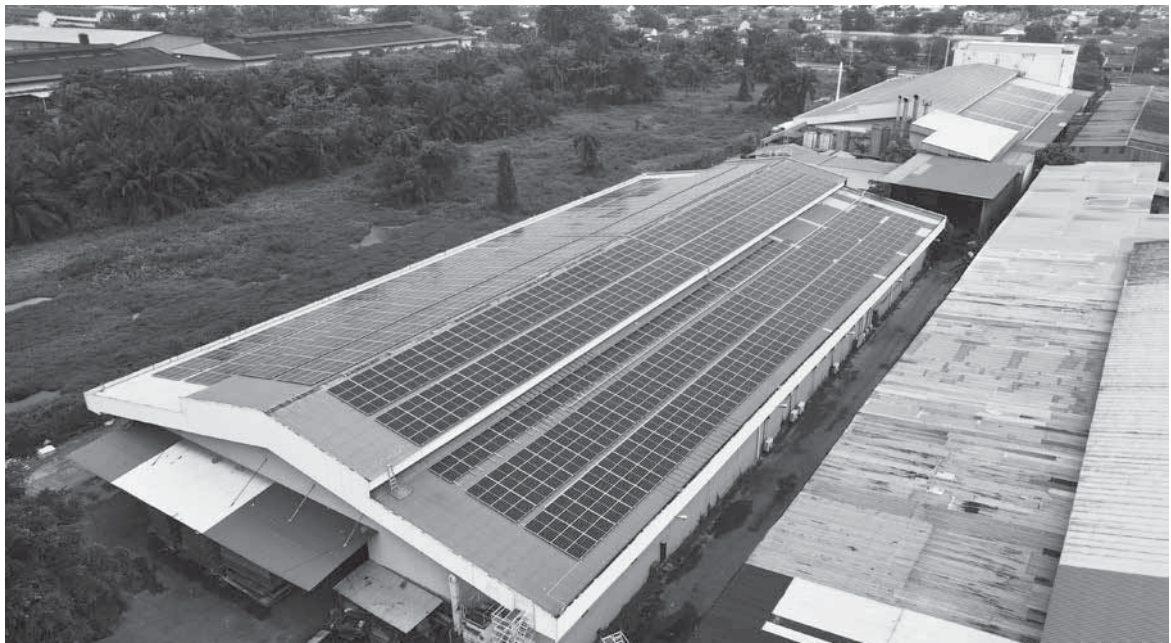
Coveright - Solar Power System
